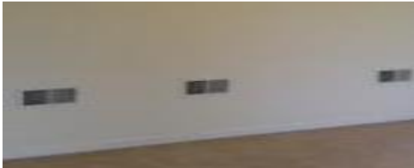
Figure 9. Air injection valves on side walls in residential houses. It can be incorporated in the design of stables with natural ventilation systems
